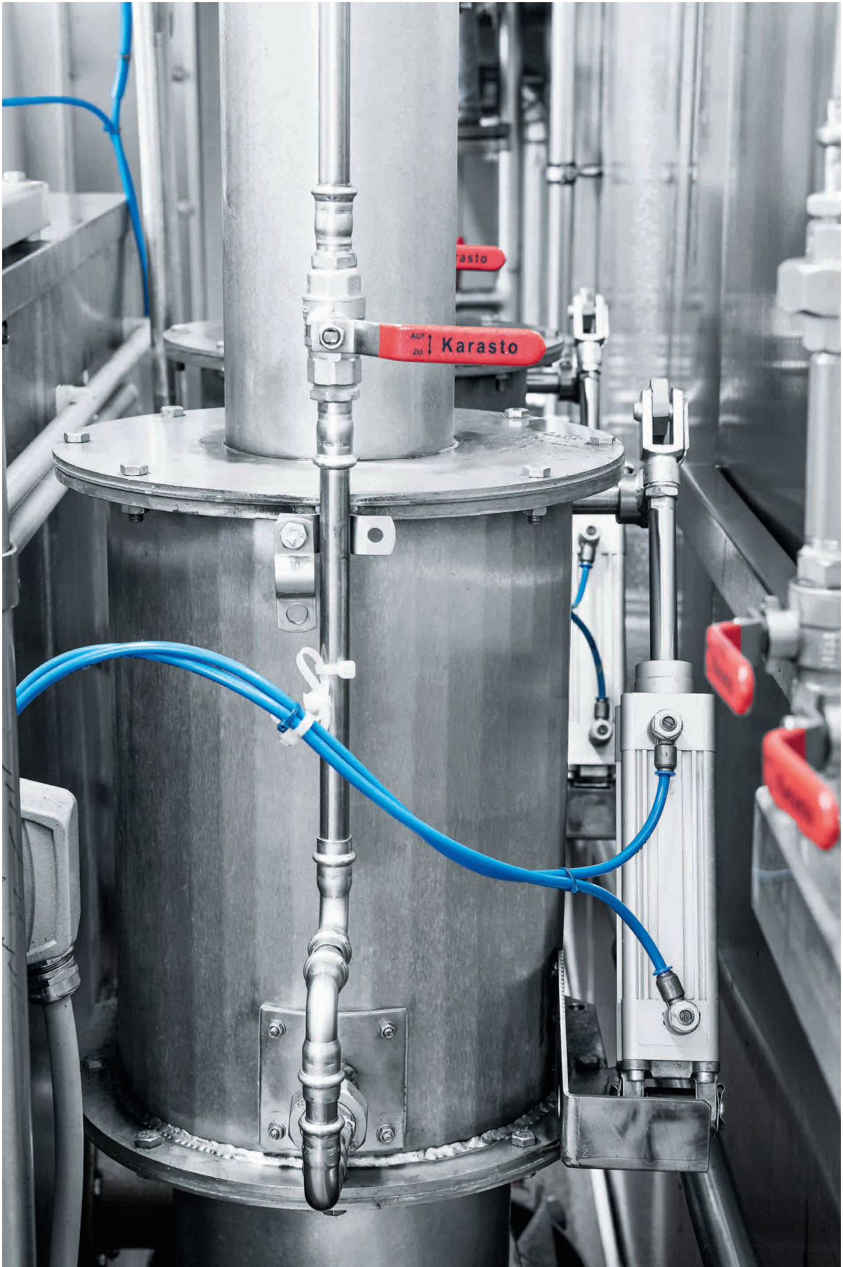
ISO cylinders DSBC with self-adjusting pneumatic cushioning PPS control the hot steam valves between the smoke generator and the smoke house.
