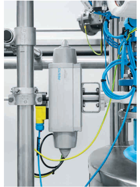
Festo quarter turn actuators DAPS control ball valves and butterfly valves on the reactor.
